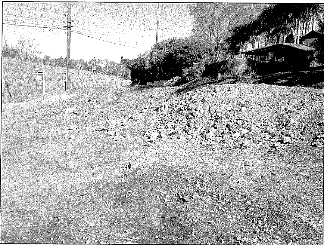
Dump fill over edge of Choya Canyon Road at Subject Properties northern intersection with Bear Valley Parkway.
