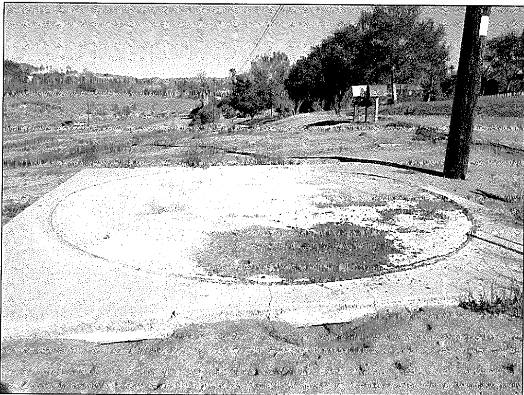
Concrete slab with remnant steel ring reportedly the location of a storage tank used to contain Oil. Dimensions 8' h x 12' diameter.
